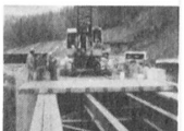
VICTORIA ISLAND Bridge. Deck replacement with prestressed wood panels. Ontario Hydro Ottawa, 1984.
