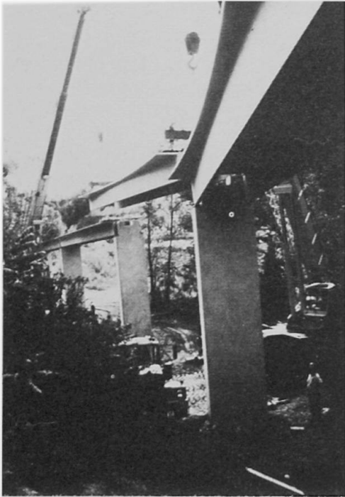
Figure 4 The Metropolitan Toronto Zoo Guideway used precast concrete double tee beams to achieve a low-cost guideway system. A cast-in-place topping provides continuity and steering curb. (Photo by author)
