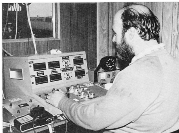
Fig. 7 Remote Control Panel.
