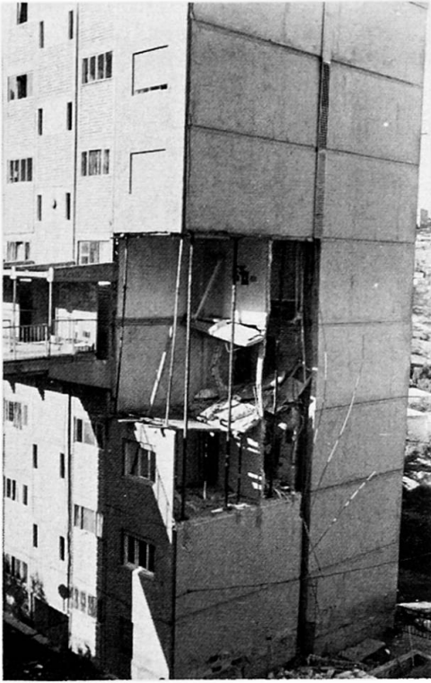
Figure (4) Results of boiler explosion in Jerusalem
