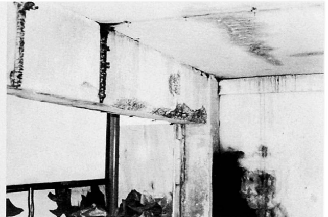
Fig.7 Spalling at the beam
