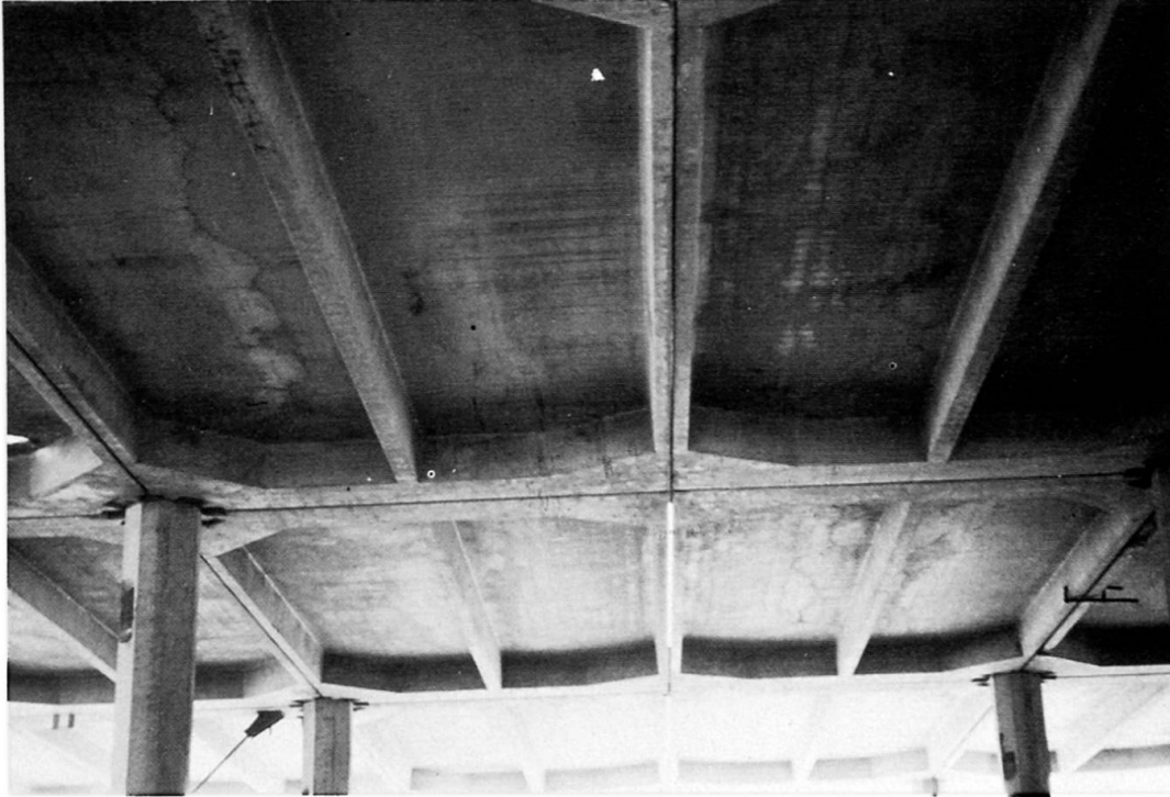
Fig 1 : Bottom view of slab elements. At the center of the span, the joint where the elements are coupled is visible.
