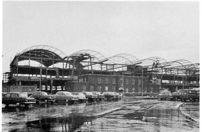
Fig. 8. The external view of seven barrel vaults built for the Port of London Authority
