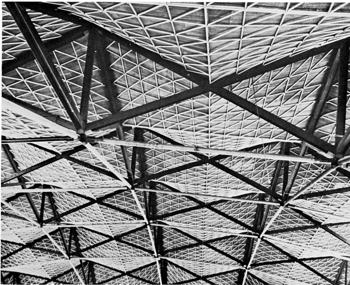
Fig. 12. Space grid roof over the Olympic Games Sports Palace in Mexico City
