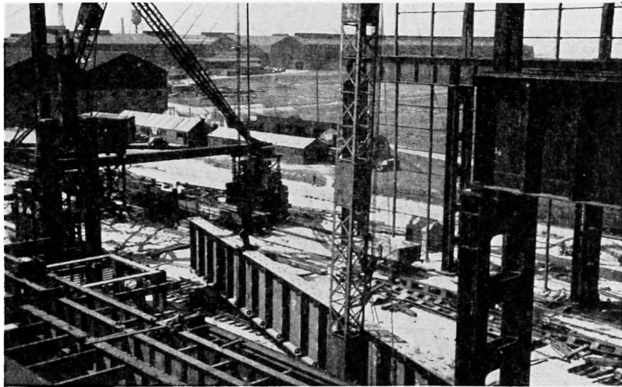
Fig. 10. 100-ton welded girder being lifted by a derrick crane and a derrick mast
