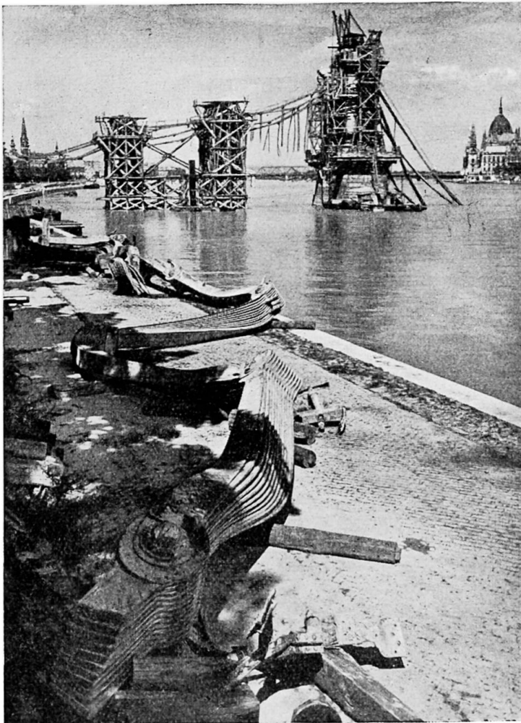
Fig. 9. Recuperated, crooked chain-bundles in foreground, supporting and staging, with the saved chain-line of the right span to be readjusted in the background.
