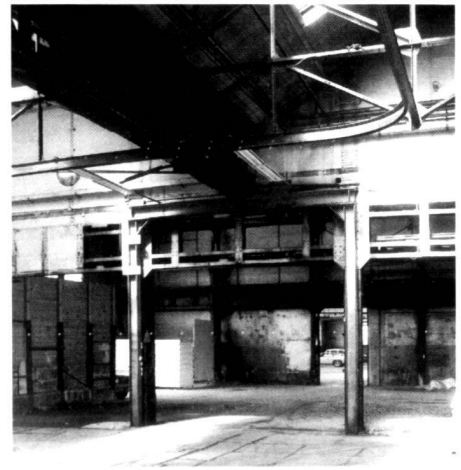
The planning site is rich in evidence of the industrial past. It is planned to allow this to survive in fragmentary form as traces in the future park.
