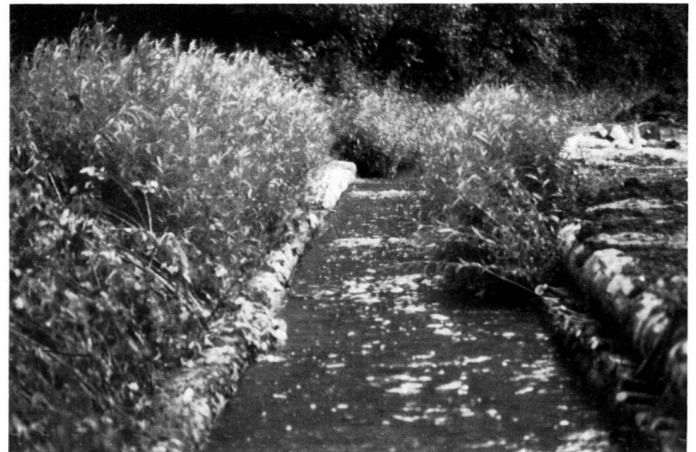
5 Left, layer of leaf blade with pine trunks to secure the base; right, 2 pine trunks with a layer of bush in between.
