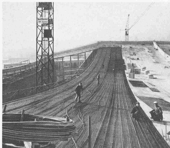
Bild 14. Armierung und prestressing steel for a 10 m wide strip of the suspended shell Reinforcement and prestressing steel for a 10 m wide strip of the suspended shell
